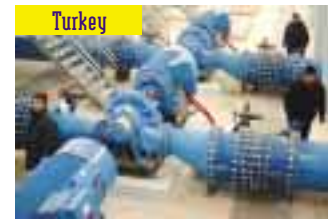
Turkey Three City Municipality Fresh Water Pumps 3300V / 300A
