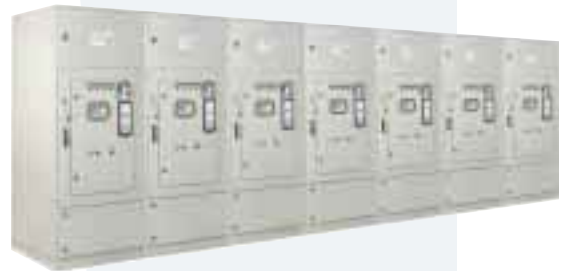
Medium voltage MCC lineup with load make fault break switch, fuses and a protection relay.
