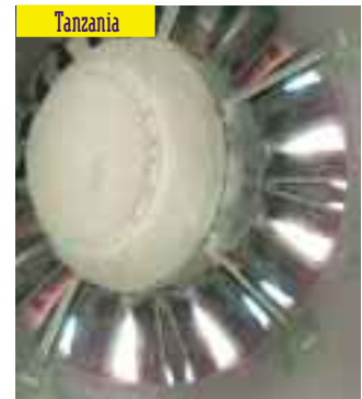
Tanzania Four Air Supply Fans in a Gold-Mine 6600V / 300A
