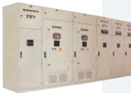
Single supply with two redundant soft-starters, where any starter can start any of the three fire extinguishing pumps 3.3KV, 110A
