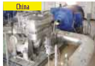
China Liquid Gas Booster Compressor 6600V / 600A
